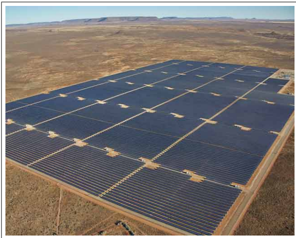
Figure 1: Aerial view of the 75MWp plant at Kalkbult. Photograph Courtesy of Eric Miller, Scatec Solar [16]
